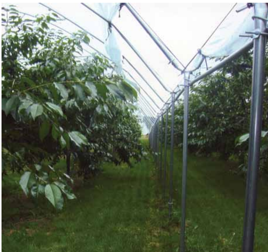
During the spring of 2009, the family decided to cover 1.5 acres of sweet cherries with a high tunnel structure. Contributed photo
