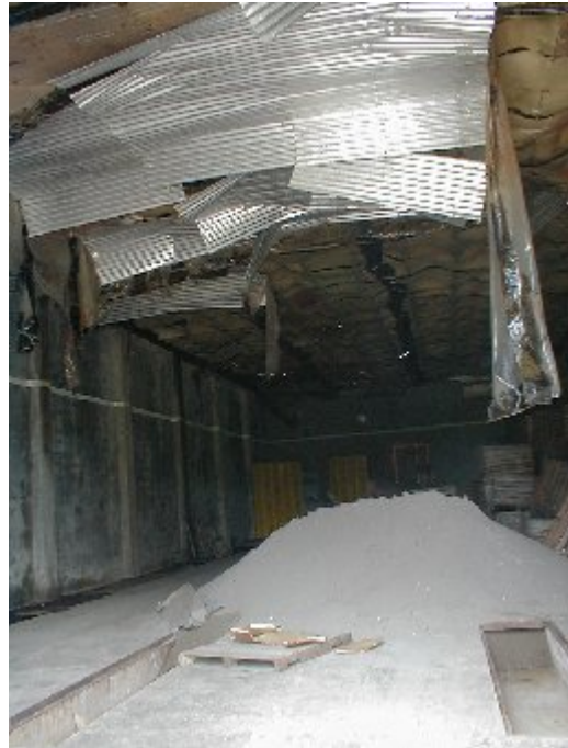
Section of building which will need extensive roof repair.
