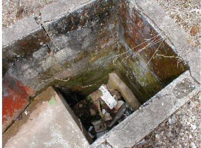
Continuation of storm drain filled with solid waste. This drain appears to lead to the road below.
