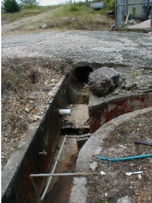
Section of existing drain between the CPGCA packinghouse and Belle Tropics packing house on property. This appears to be a storm drain into which effluent (grey water) from both buildings drain. CPGCA building is to the left.
