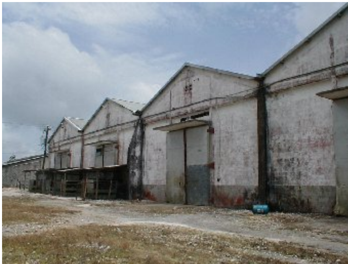
Side view of CPGCA warehouse showing exterior of the smaller bays. Covered under sheds are the forced air compressors currently in use in the functional bays. Note mould on walls.
